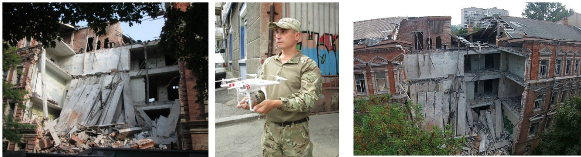
a b c Fig. 2. Using a UAV to inspect the destruction of a building (Dnipro, 2012): a – house, 25 Artema Street; b – UAV operator; c – UAV video recording
