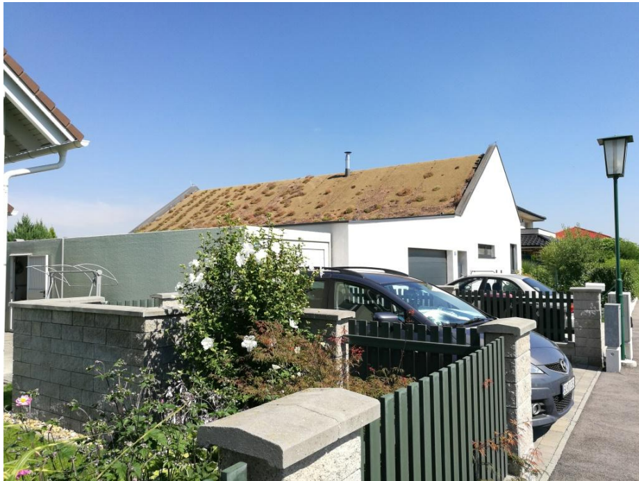
Fig. 1. Failed extensive roof greenery
