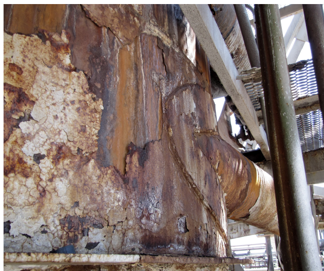
Fig. 2. Corrosive wear of the chimney trunk over 30%
