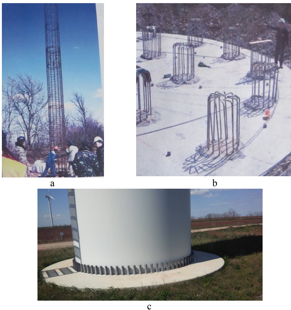
Fig. 4. The construction site of the wind power plant-65: a, b – setting of frameworks of piles; c – prepared foundation
